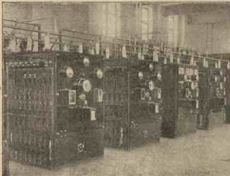
The power panels at the great Post Office Wireless Station at Hillmorton, near Rugby.
