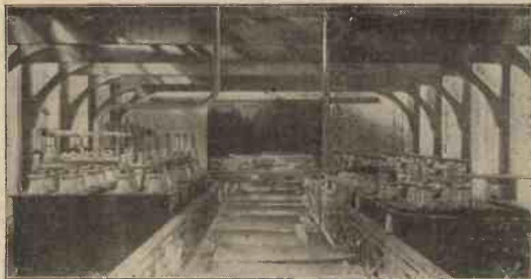
Some of the big condensers in the inductance room at the Rugby Station.
